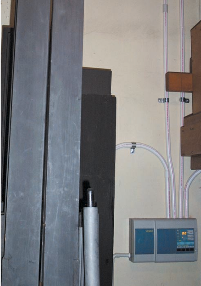
VESDA control panel and sampling tubes in the organ chamber
